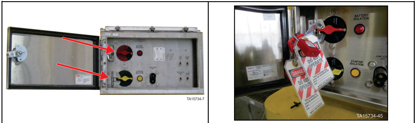
Battery Isolation Box – Battery isolation switch in OFF position with locks in place
